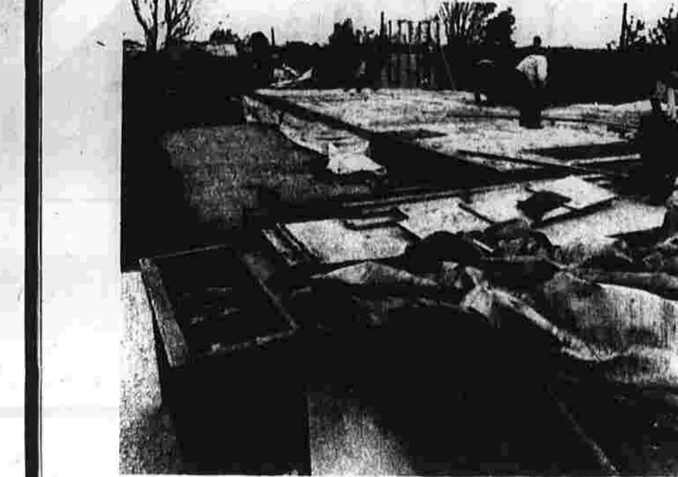
Workers on the James Woble home in Windsor Locks, pull out all the nails from the ground floor and will start in a few days to rebuild. The record player in foreground was silent being battered by the tornado which hit the Route 75 area Wednesday. (UPI photo)
